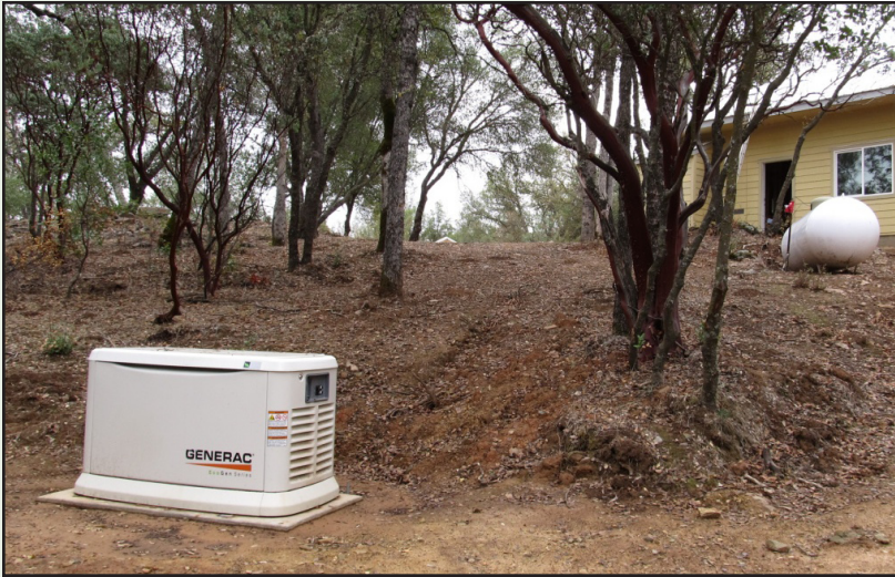
Propane-Powered Backup Generator and Tank
