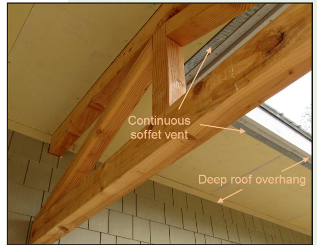
Continuous Soffit Vent and Deep Horizontal Roof Overhang
