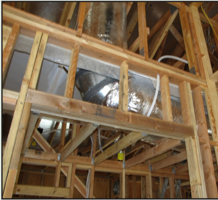
Main Air-Return Duct (concealed, but still in the conditioned space)
