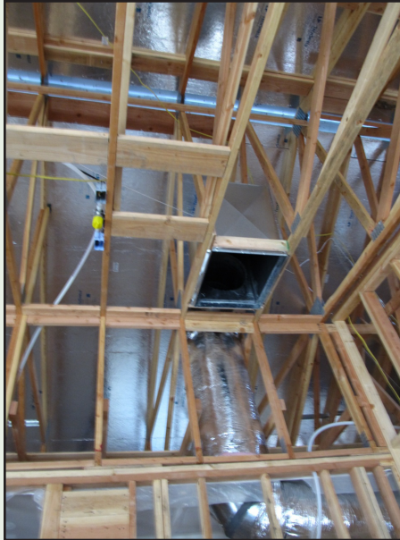
Air-Return Vent and Duct (Great Room)
