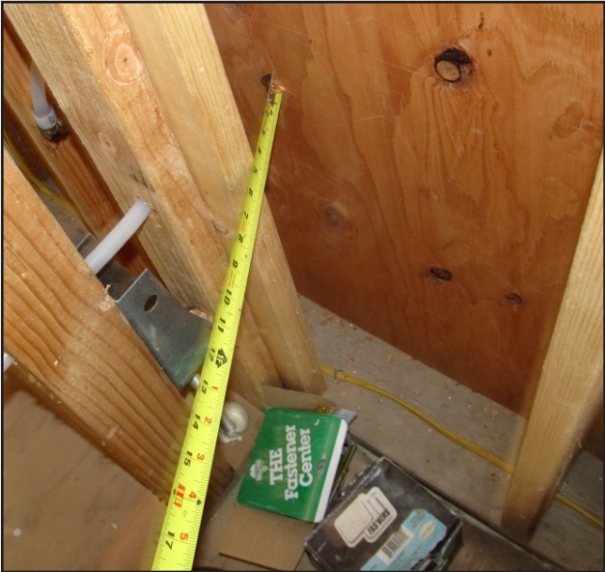
Gap Between Interior and Exterior Walls
