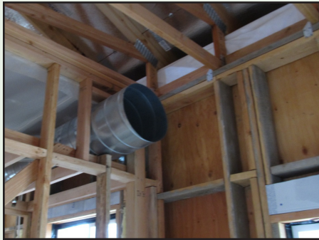
Duct Into Bedroom
