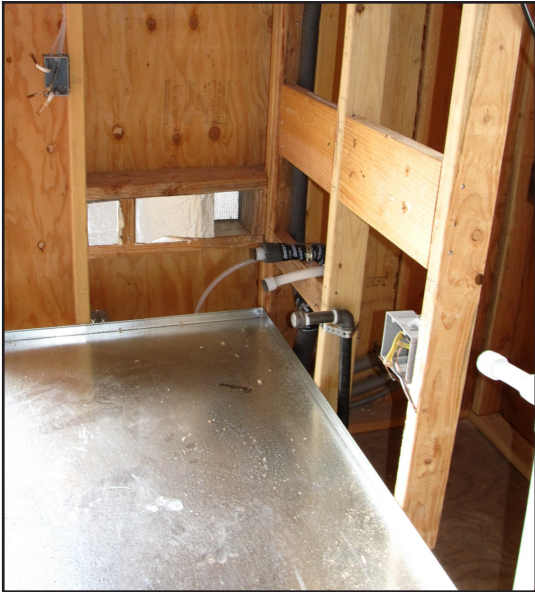
Site for Combined Hydronic Heating System and Energy-Recovery Ventilator
