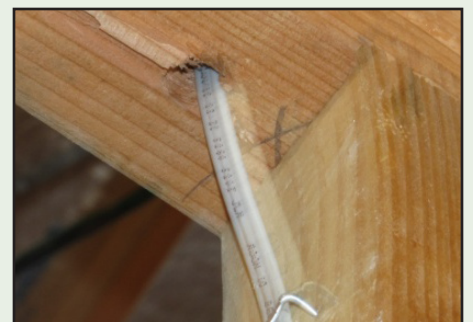
Hole for Electrical Wire (to be sealed)
