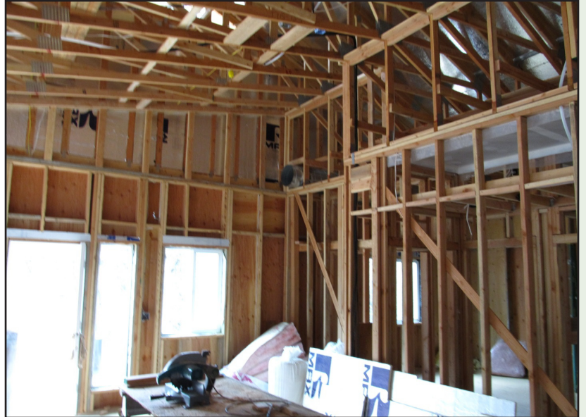
Duct Into Great Room and Site for Wood-Burning Stove
